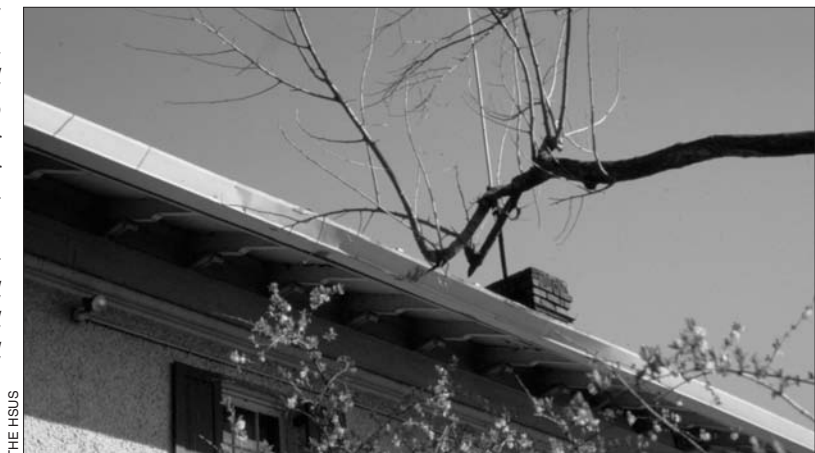
Figure 87 This branch is a virtual highway to the roof for squirrels. After repeated invasions of the building, the branch was finally trimmed back and squirrel traffic rerouted to nearby trees.
